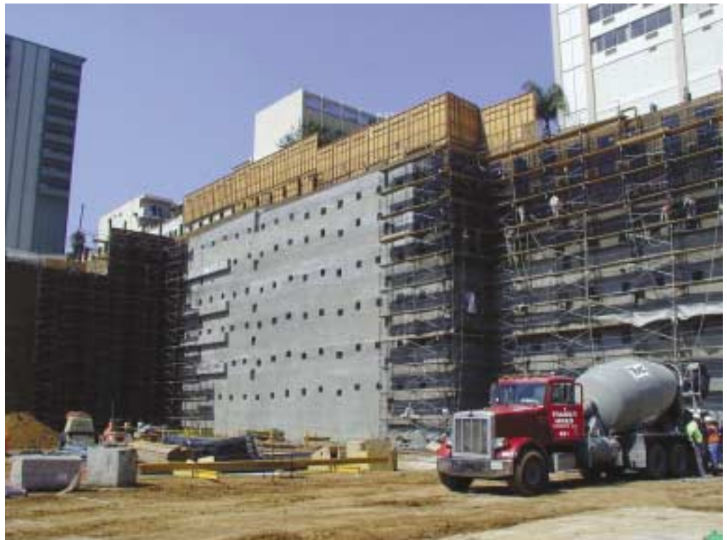
Partially completed Hollywood & Highland project in Hollywood, Calif. This project required over 13,000 yd 3 of 25-in.-thick shotcrete walls. A section of sawcut preconstruction panel for the project showed complete encasement of the reinforcing steel, even with lap-spliced #11 bars
